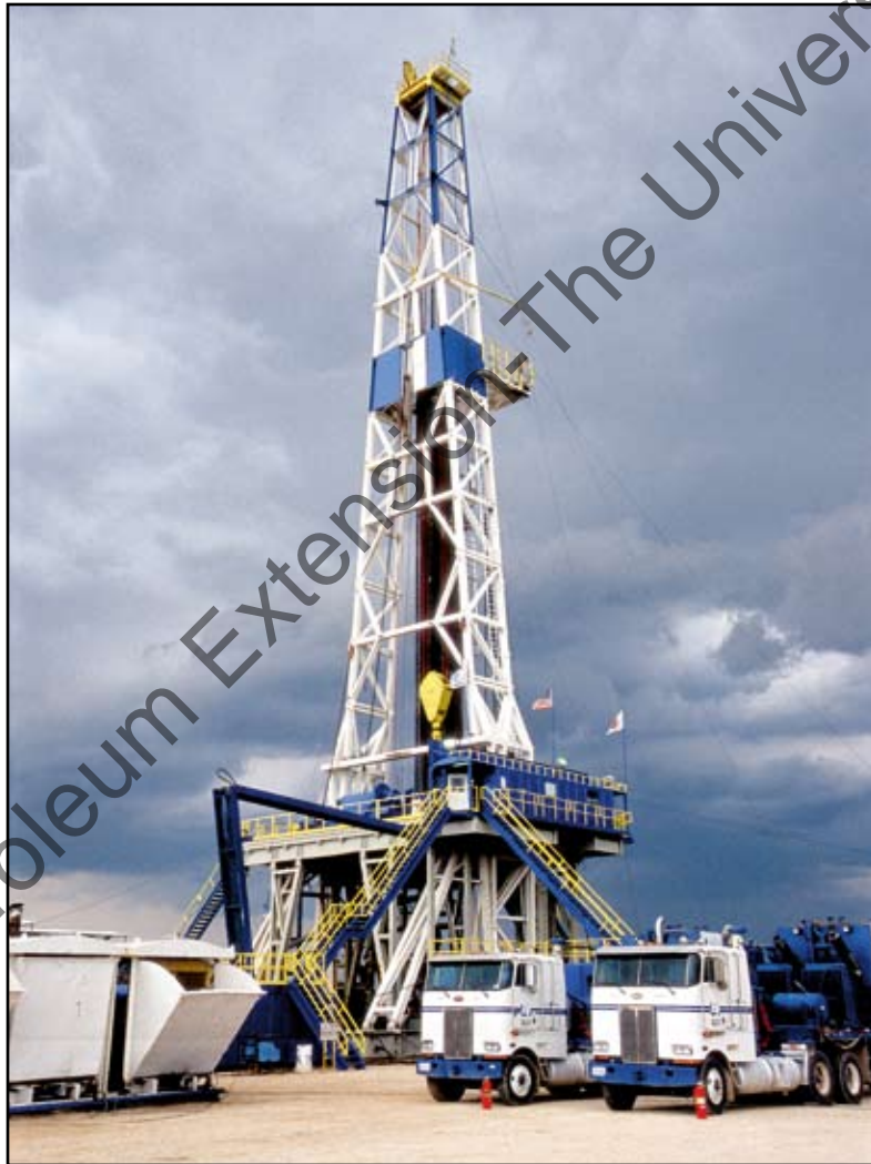
Figure 1. Drilling rigs are large to accommodate the size of the drilling equipment and pipes.
