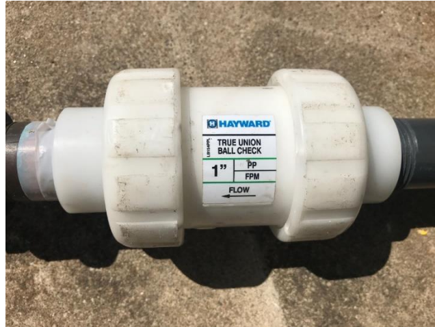
Figure 10 - Water Pathway Check Valve
